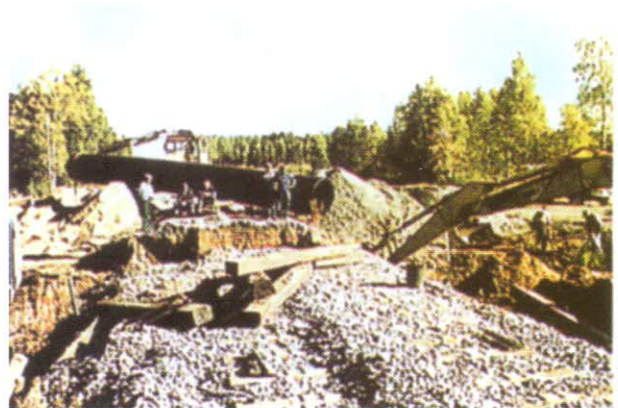
Kaskö, Finland; Culvert under railway. Open cut renovation finished in 3 hours. Dimensions 1200 mm – 1600 mm.
