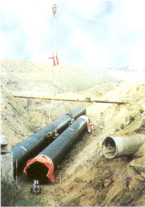
Wolfen, Germany; A parallel, 2 x 1400 mm ID industrial waste water pipe-line. Total length 2046 m.
